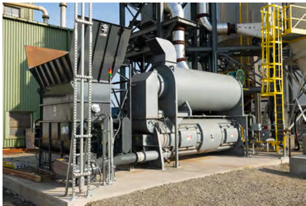
Feed Ash Dryer
